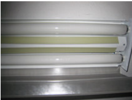
Fluorescent light fixture with glow strips installed
